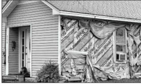
A dog sits Thursday on the front porch of a home in West, where the siding has been melted away by a fire from the house next door. The fire followed the explosion of a fertilizer plant Wednesday night. RODOLFO GONZALEZ / AMERICAN-STATESMAN
